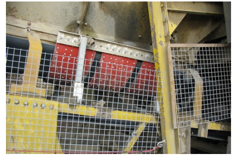
Cement works - 600 tons per hour 1.000 Belt
