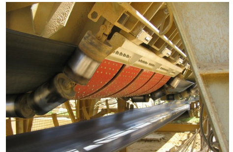
Cement works - 800 tons per hour 1.200 Belt ( 5 hanging straps )
